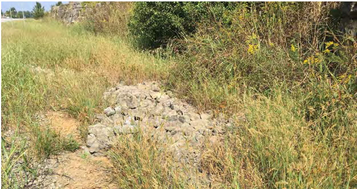
Sinkhole repair along KY 245@ MP 6.1-6.2.
