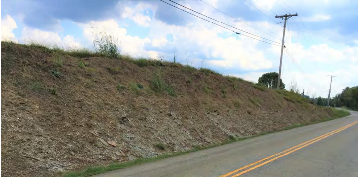
The New Albany Shale Formation exposed in cut slope along KY 733 @ MP 11.9.
